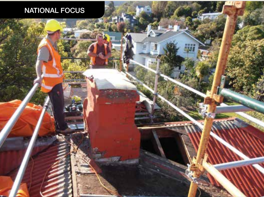
Chimney stabilising work at Category 1 Historic Place Melrose House (CREDIT: NELSON CITY COUNCIL)
